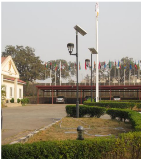
Fig. 1: A Photograph Some of the Solar Powered LED Street Lighting Systems at AUST.
